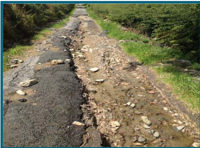
Road Pavement Erosion
