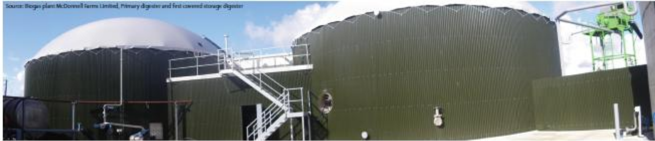
Source: Biogas plant McDowell Farms Limited, Primary digester and first covered storage digester
