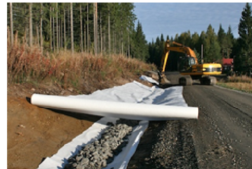
Drainage improvement – always!
