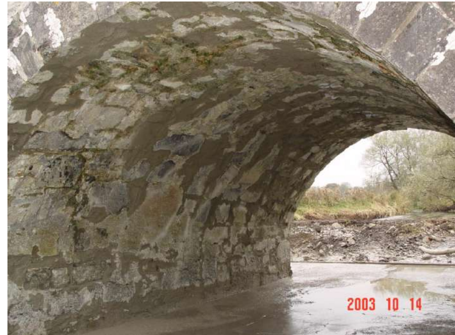
Stabilise foundations, protect against scour, pressure point arch and install tie bars and pattress plates
