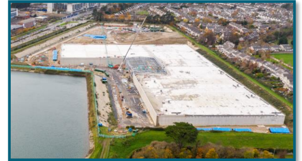
Photo: Stillorgan Covered Reservoir, from Uisce Éireann
